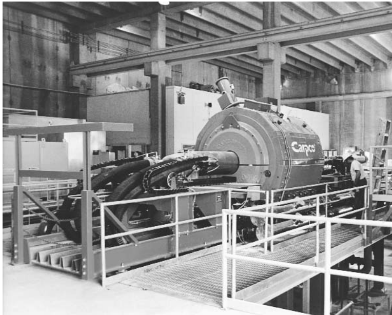
FIG. 19-54 Superconducting magnetic separator operating in a kaolin treatment plant. (Courtesy Carpco, Inc.)
